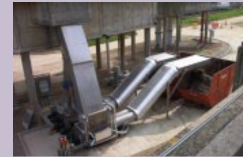
Crawley STW, 18m 3 /hr capacity system
