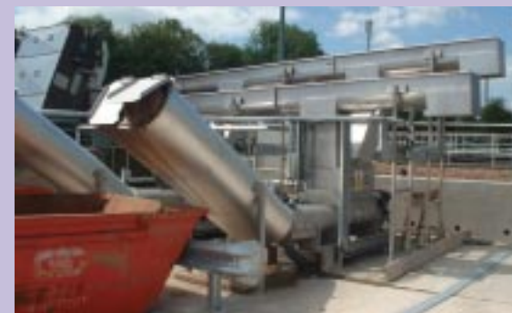
Severn Trent Water, Barnhurst: Turnkey screenings handling system
